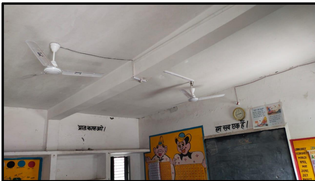
Pic 10: Fans installed in the classrooms of PS; Rauniya donated by Pragarth
